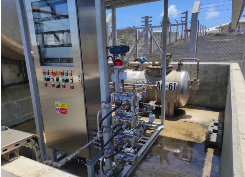
Ascension new additive dosing rig
