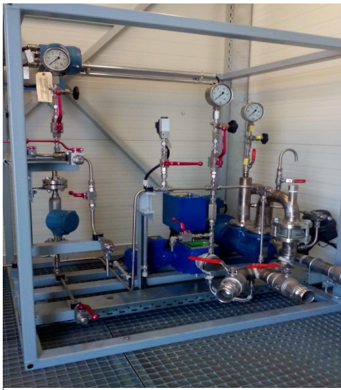
Fig. 1 DRA additive skid system
