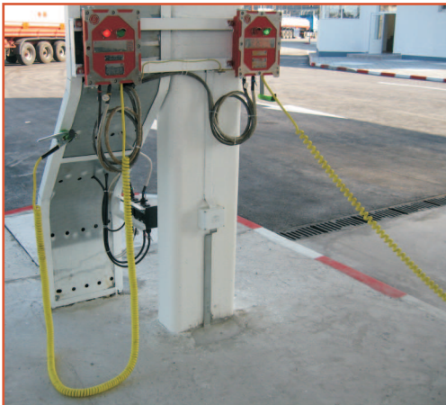
Two of EGT4 with coiled sensing cables
